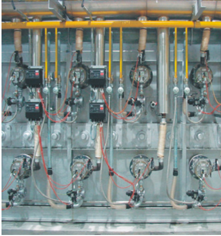
Roller hearth furnace
