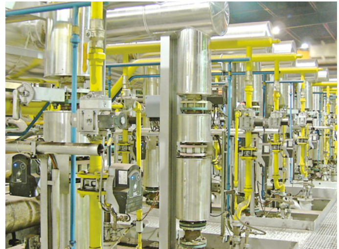
Walking beam furnace with overhead firing
