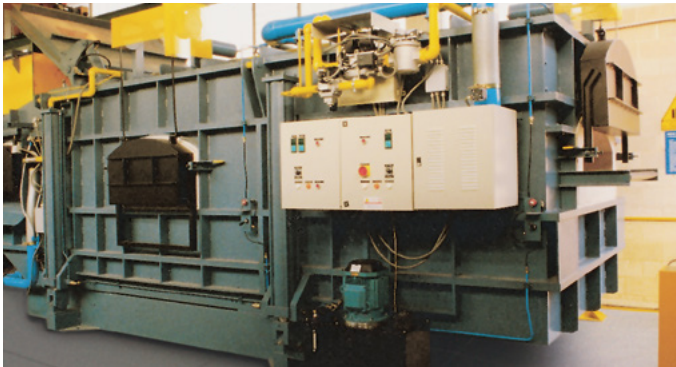
Air/gas ratio control on melting furnace for ensuring stoichiometric combustion over the entire capacity range
