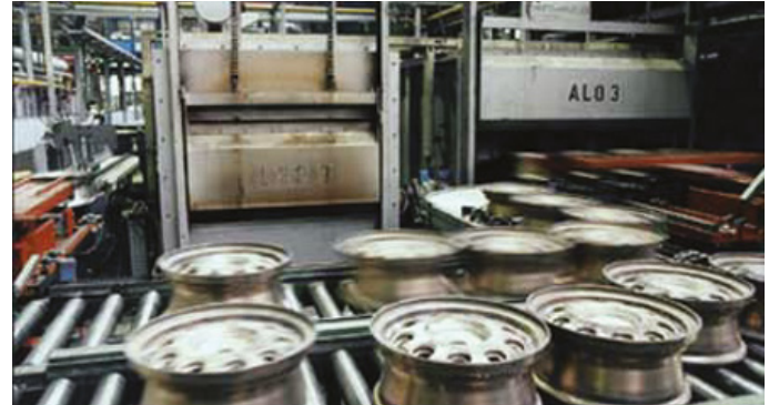
Aluminium age-hardening furnace with air/gas ratio controls for low air pressure protection
